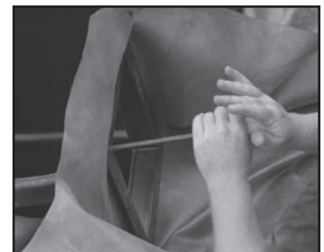
Fig. 16 Replace the skimmer liner plate and the two corner screws, and then proceed with the bottom two corners. Punch remaining holes, thread screws.
