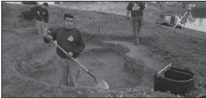
Fig. 6 Dig the pond to its max depth and finish excavation of the skimmer hole.
